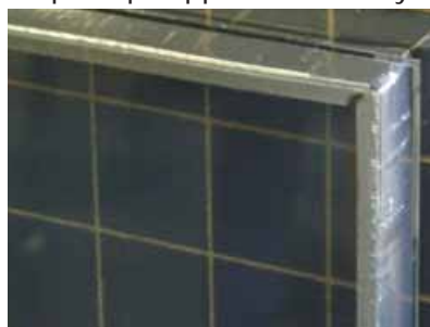
Proper Tape Application Quality
